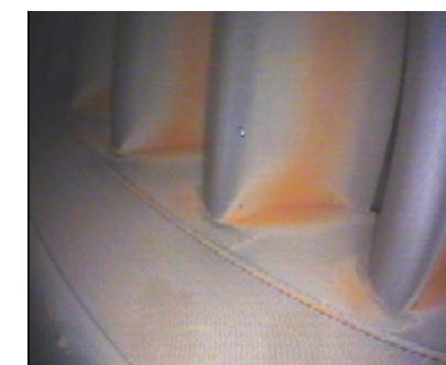
Damage of turbine without conservation
