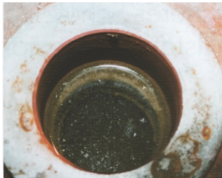
Conserved pipe section, filled with water for 8 years
